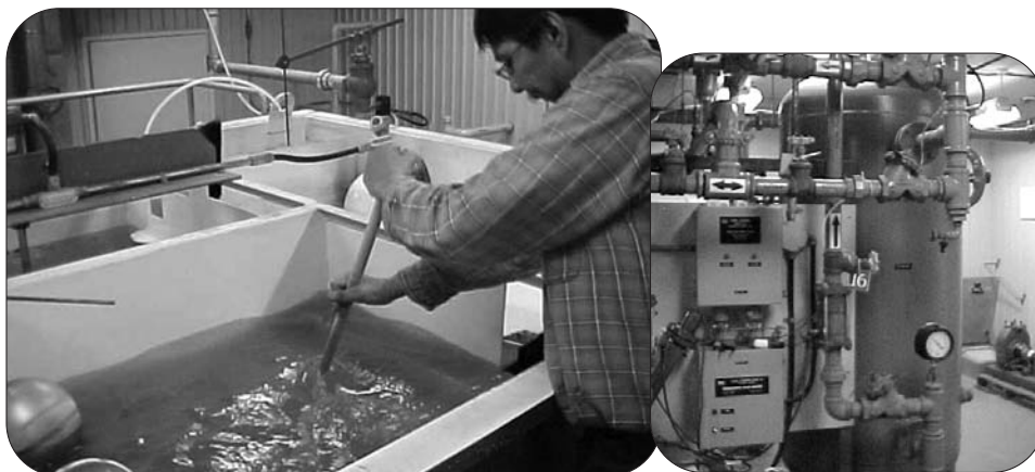
LEFT: FORT PROVIDENCE OPERATOR STIRRING FILTER BED DURING BACKWASH
