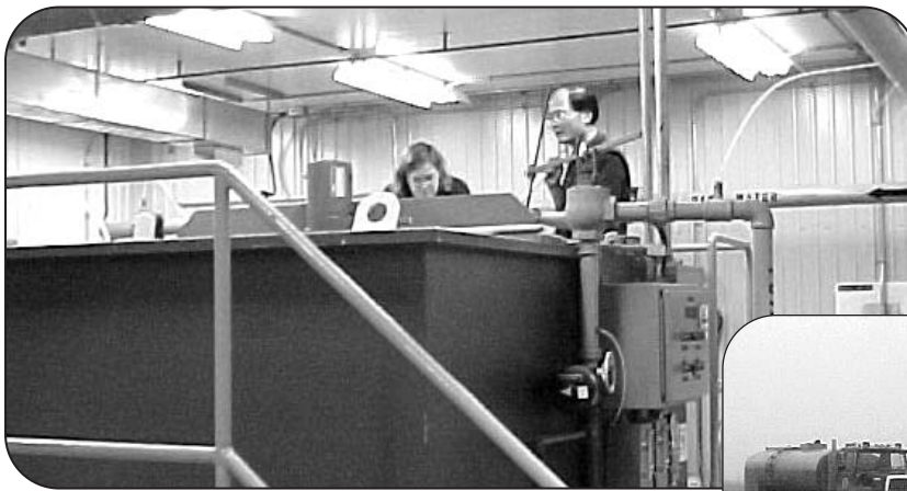
ABOVE: FORT PROVIDENCE PLANT RIGHT: FORT PROVIDENCE WATER TRUCKS
